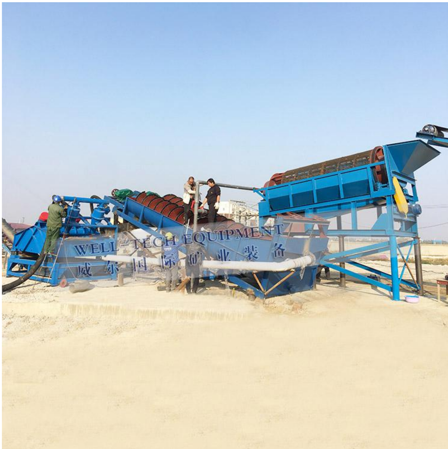
Wash Sand plant
