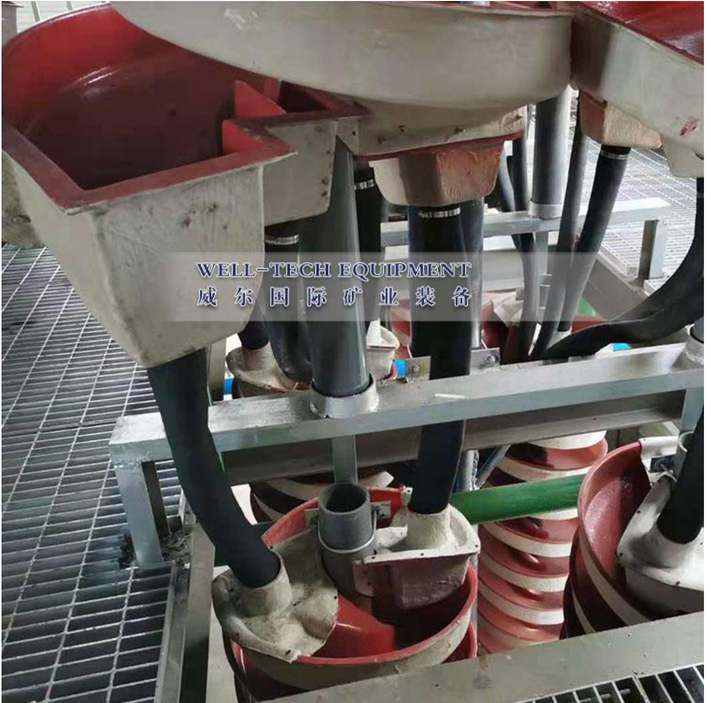
quartz processing plant
