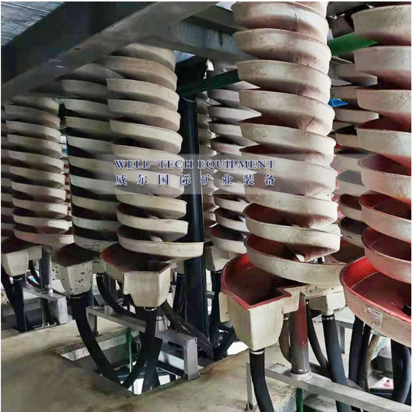
Silica washing plant in Bangladesh
